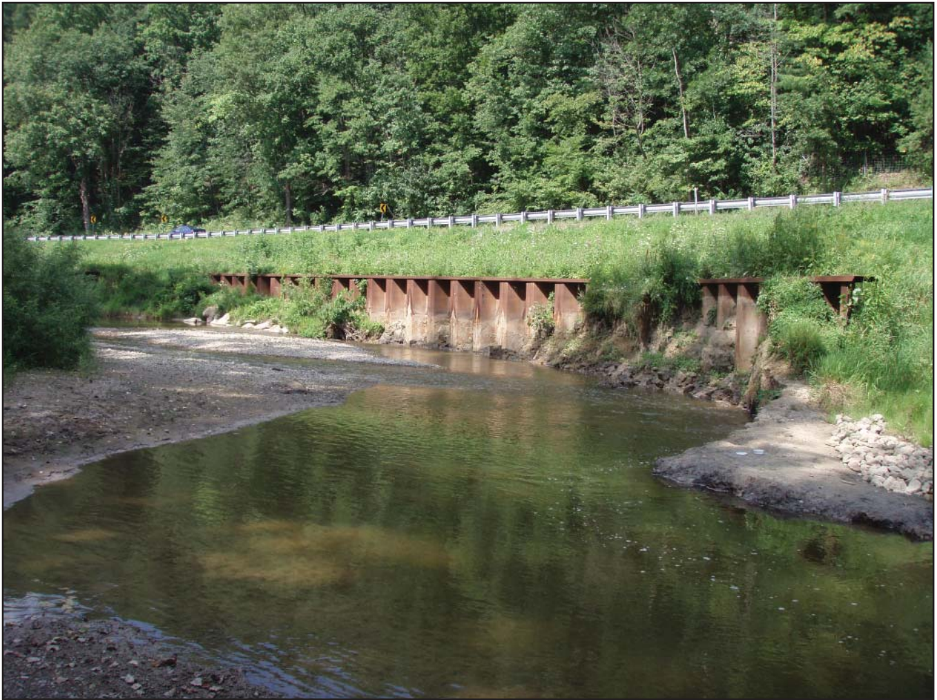
Erosion of stream bank in Mill Creek just upstream of mussel survey Site 2. The steel wall was installed a few years ago (Photo by Peter Badra).
