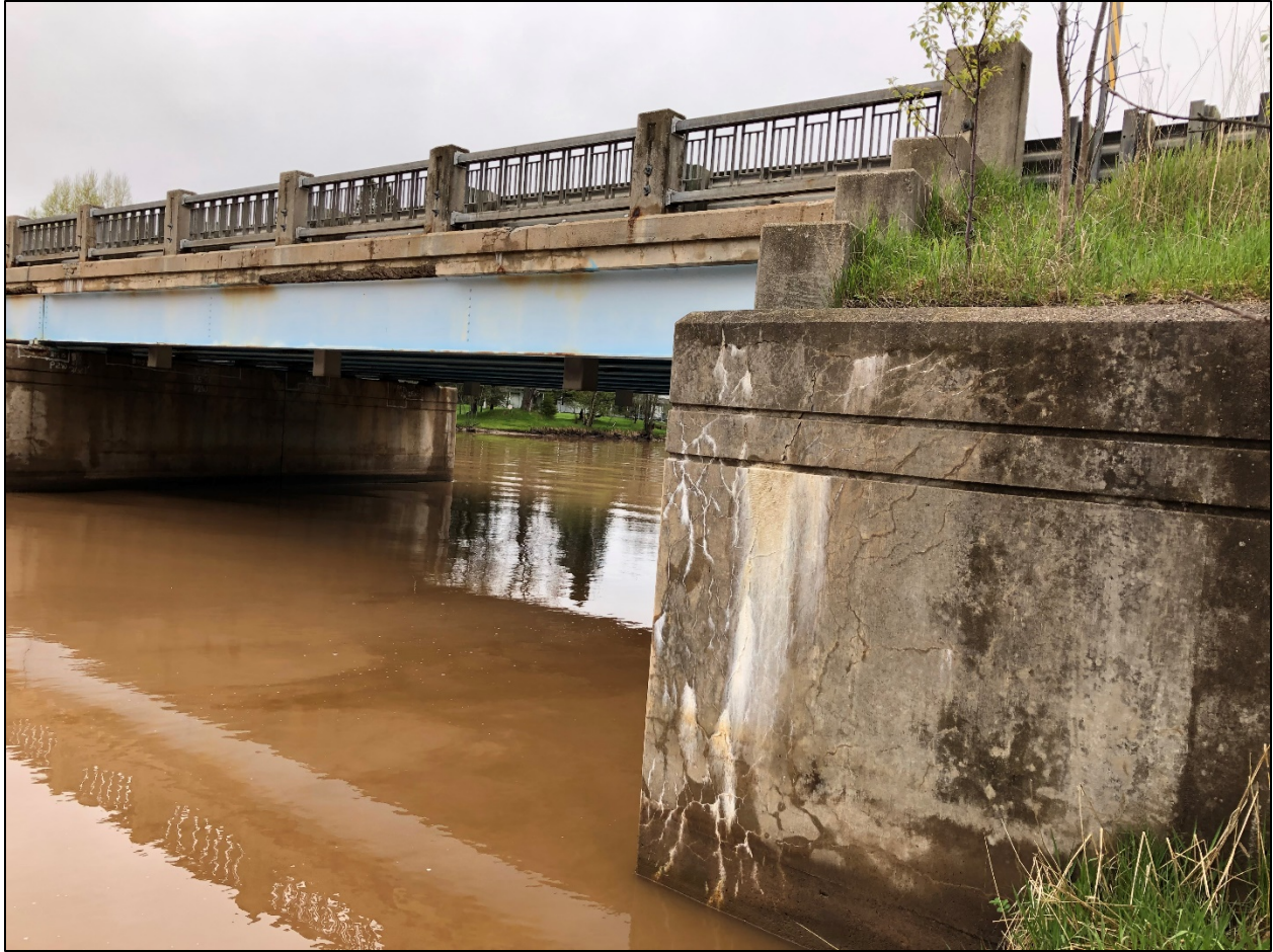
Figure 20. The condition of the M-134 bridge crossing over the Pine River is deteriorating. Crumbling concrete and cracks in the retaining wall were observed.
